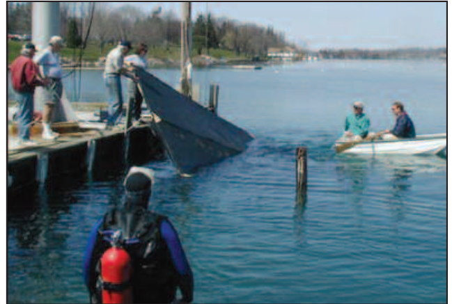
A crew on Skaneateles Lake begins to place the benthic barrier they constructed.
